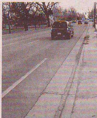
Felix Wong | for FCNow The bike line on this section of Taft Hill Road, just north of Mulberry, disappears.
